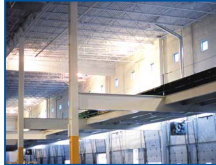
This manufacturing facility utilized K-13 for acoustical control and much needed thermal control.
