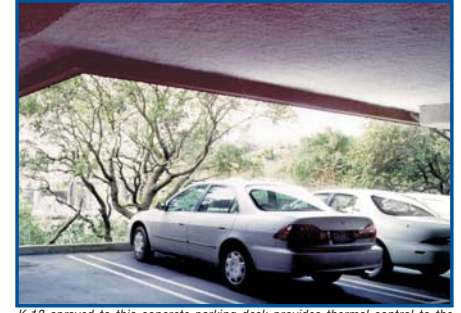
K-13 sprayed to this concrete parking deck provides thermal control to the conditioned spaces above.
